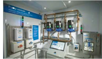
Pumping Booster pump system demo
