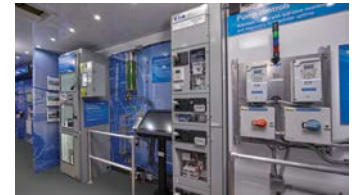
Process industry MCC and 18-pulse variable frequency drive demonstrations
